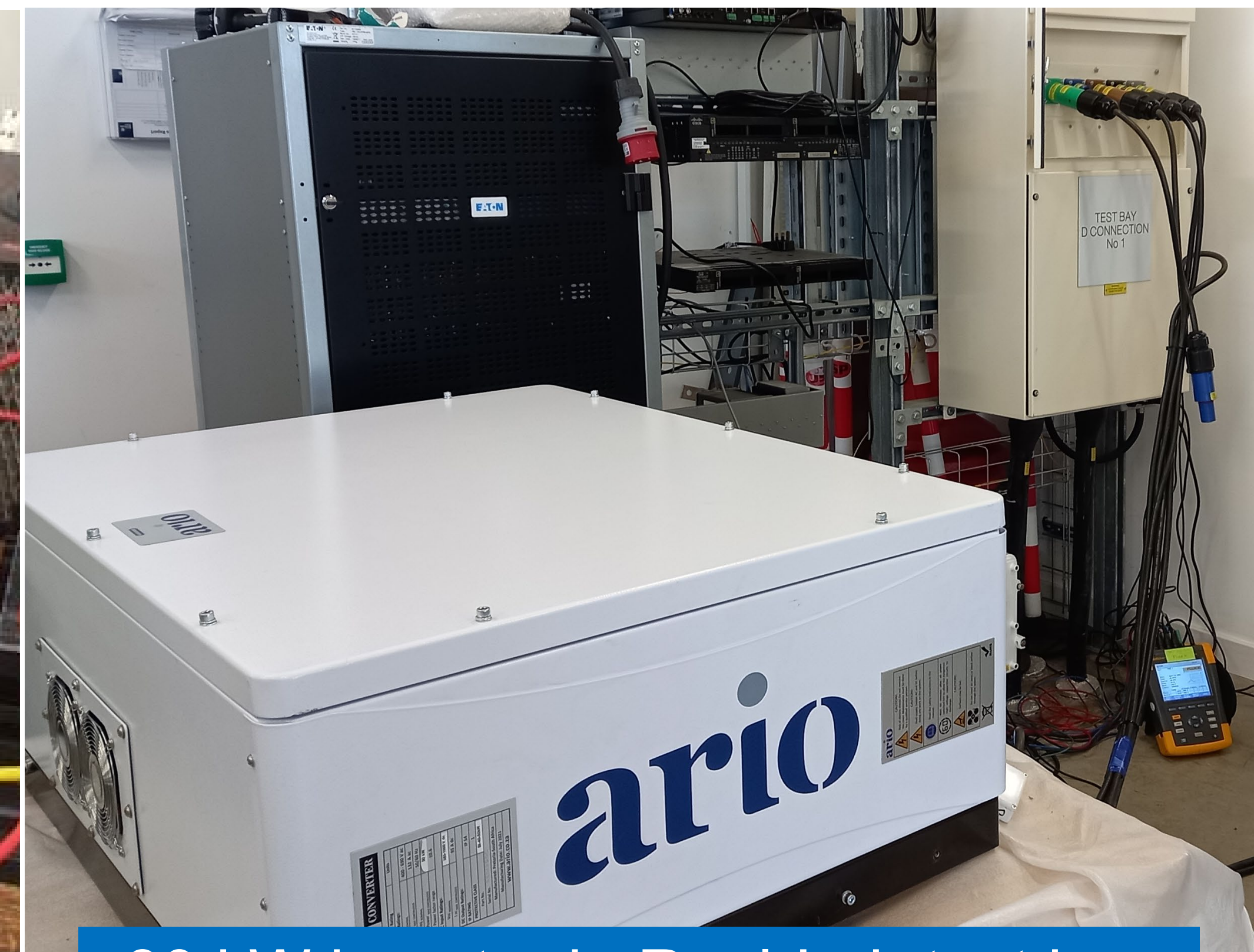
80 kW inverter in Real-Lab test bay
