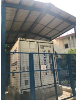
Socomec BESS 200kW/274kWh
