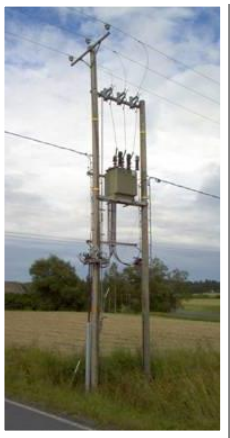
20/0.4 kV distribution substation
