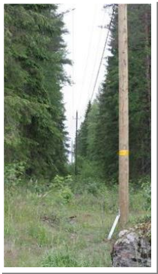
20 kV overhead line
