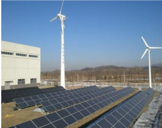
PV & Wind Power
