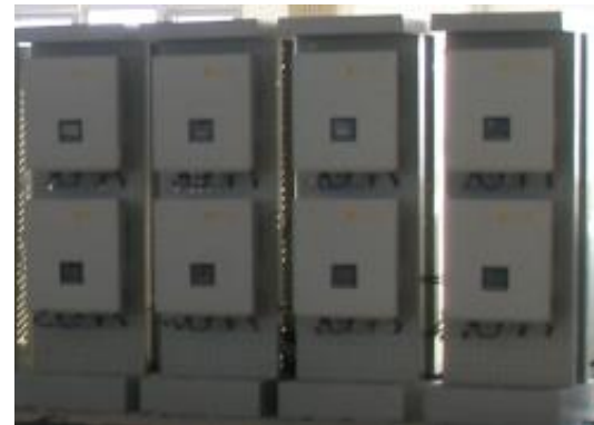
DC PV Converters
