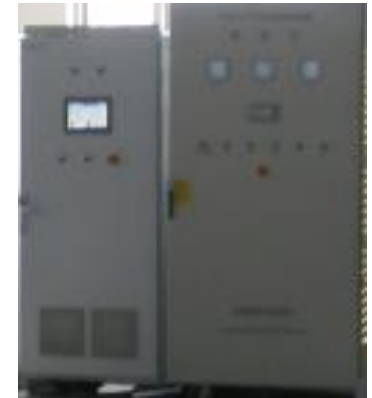
DC Wind Power Converters
