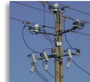
Pole Top Transformers
