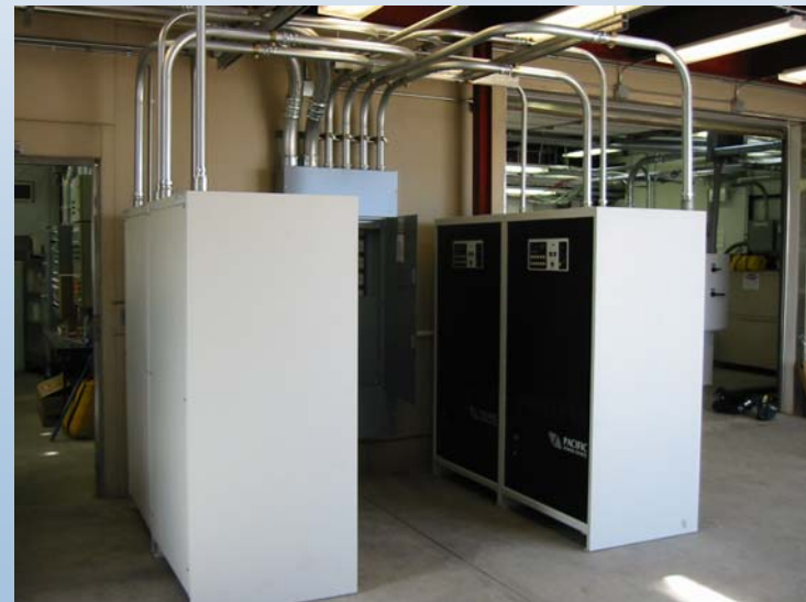
Utility Grid Simulators – Primary injection test set
