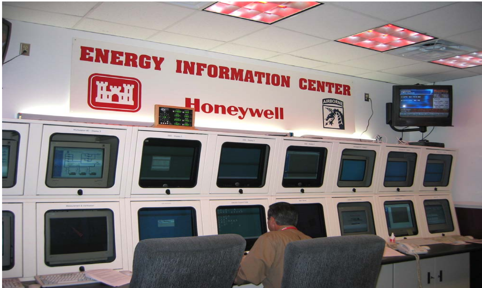
control room at Fort Bragg, NC
